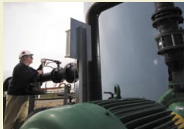
(Above) Ron Turnbull inspecting pipework and instrumentation which will receive high quality water from the Water Corporation's Kwinana Water Reclamation Plant.
