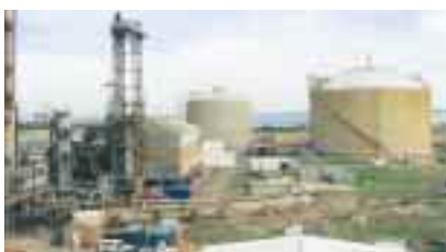
The demolition of the vetrocoke section of the 32-year-old ammonia plant at Kwinana.
